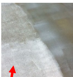
Structured surface (coarse „orange skin“) after the tackifier has been applied with a coarse-pored foam roller and dried off completely.
